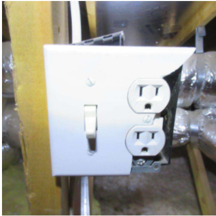
Image 3.4.1 Broken Outlet Cover
