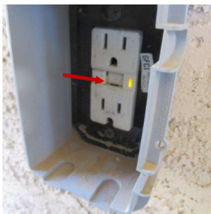
Image 3.3.2 Broken GFCI Test Button
