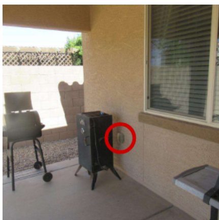
Image 3.3.1 Broken GFCI Location
