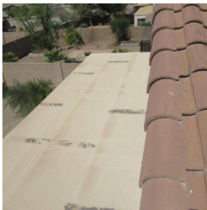
Image 2.2.2 Peeling coating from joints on patio roof
