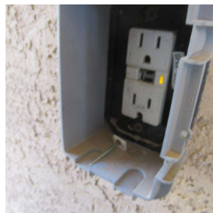
Image 3.3.3 Broken GFCI Test Button
